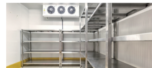
RESTAURANT COLD ROOMS
